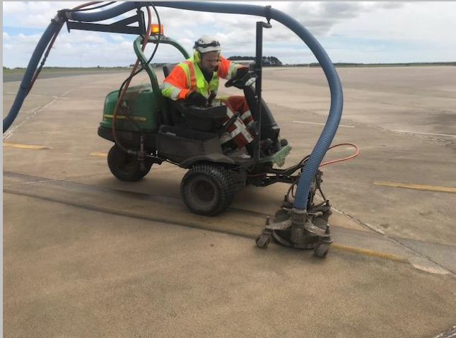
Satellite Hydro-Blasting Unit
