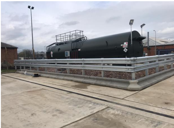
New operational fuel tank
